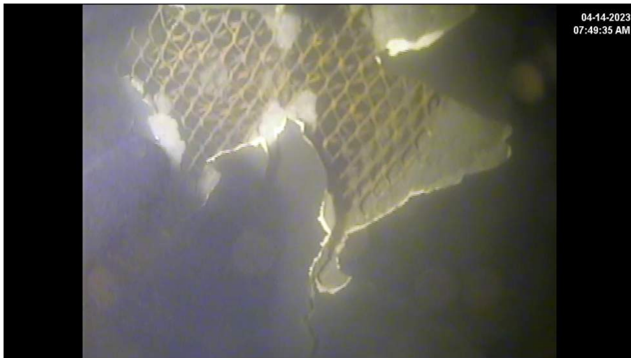
Photo 3 – F14 – North Face – 10 feet below surface – Vessel debris abutted to pile
