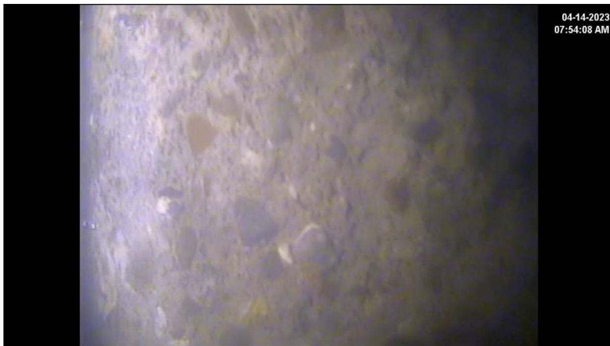
Photo 4 – F14 – West Face – 2ft square section is sheared off 4 feet below the surface.
