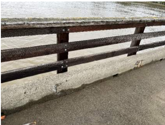
Photograph 9: Concrete cracking at bull rail
