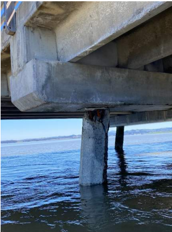
Photograph 5: Severe damage at the top of Pile F14
