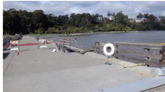
Photograph 10: Broken wood railing
