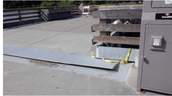
Photograph 8: Damaged expansion joint cover plates
