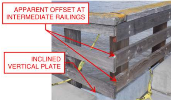
Photograph 7: Lowered northwest end of causeway
