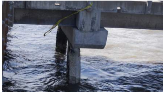
Photograph 4: Pile shifted from support
