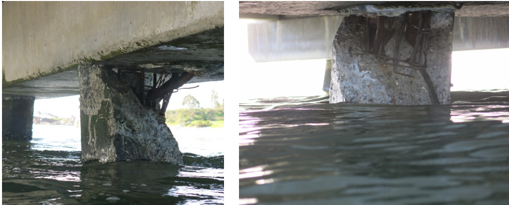
Figure 2: Damage at Pile F14, Bent 14 Northern Pile
