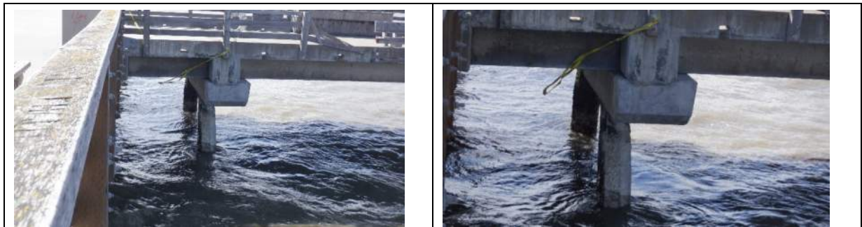
Photographs 8 and 9: Possible damage at pile-beam connections at Bent 14
