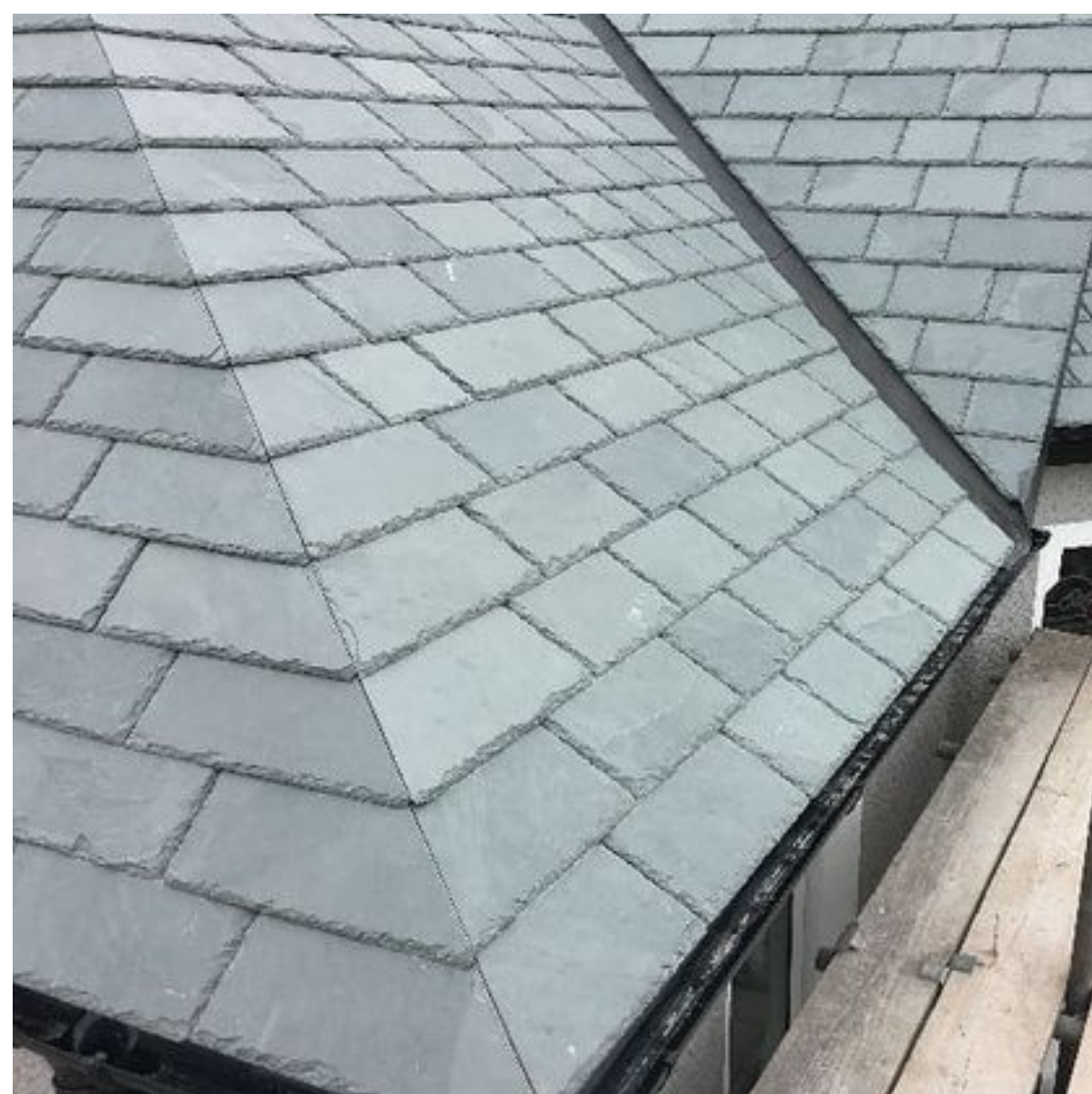
GREEN-GREY SLATE ROOFING
