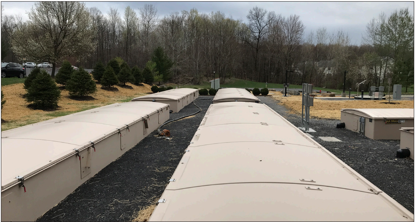
The AX-Max uses a passive, attached-growth treatment process that is inherently stable and has minimal operation and maintenance requirements. The Max also minimizes noise and odor, making it "neighborhood-friendly." (Photo courtesy of the Dutchess County Water and Wastewater Authority.)
