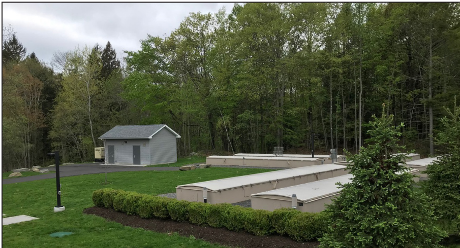
An AdvanTex® AX-Max™ Wastewater Treatment System – with its low life-cycle costs and small footprint – was chosen as the best replacement for a failing treatment plant in the community of Pinebrook. (Photo courtesy of Julie Barown.)
